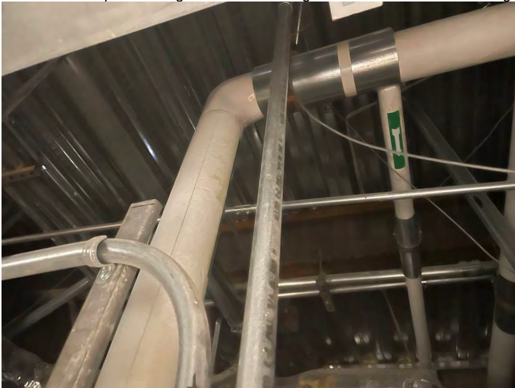
Photo 7: The pipes in the area are insulated with fiberglass with PVC fittings. They are not expected to be impacted by the project.
