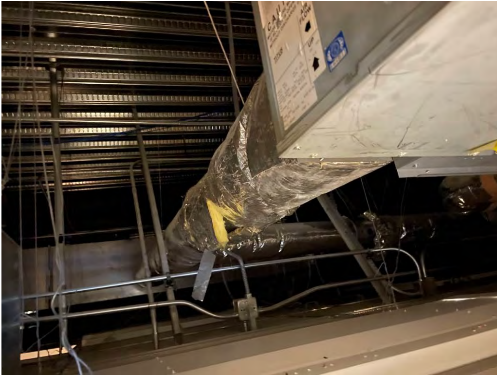
Photo 5: Bare metal pan decking and assorted hangars observed above the ceiling.
