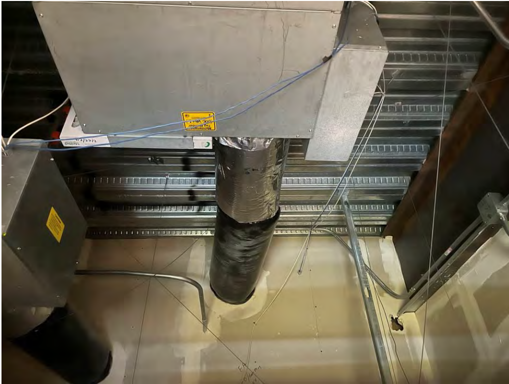
Photo 3: Non asbestos containing duct insulation and un-textured GWB system that is less than 1% asbestos when composited (GWB, joint compound, tape).
