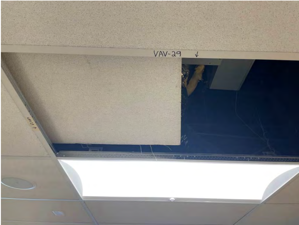
Photo 1: Typical VAV box locations were identified on the suspended ceiling t-grid. The ACT is negative for asbestos.
