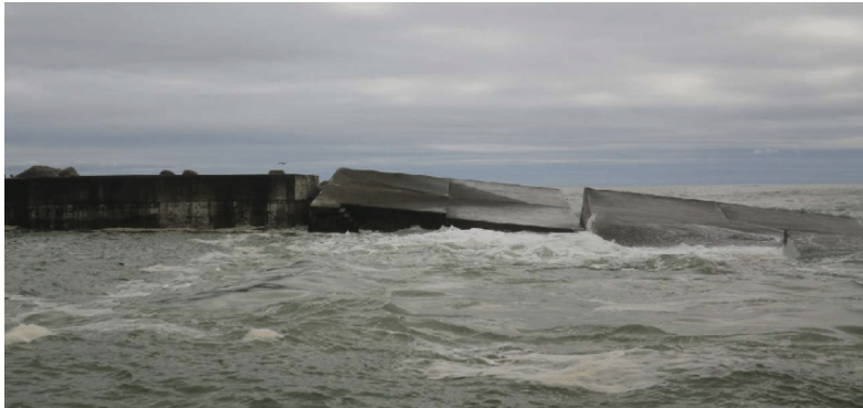
Figure 41: Breakwater failure in Japan after 2011 Tohoku Tsunami.
