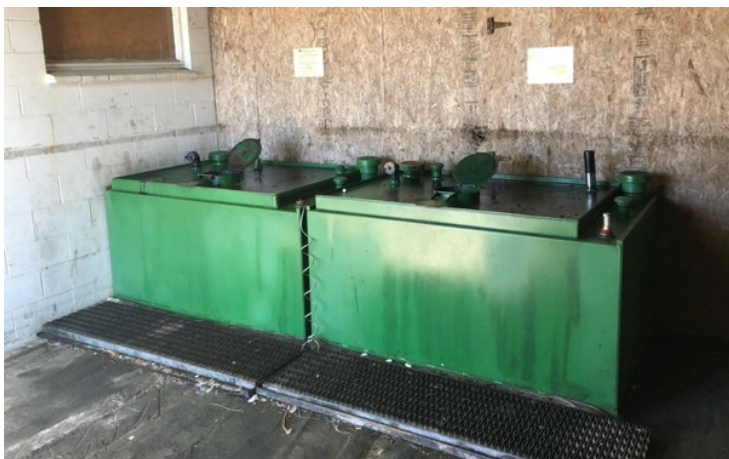
Figure 35: Chemical storage tank in Westport Marina.
