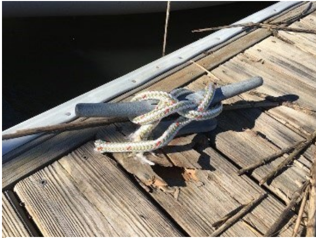
Figure 36: Cleat ripped from dock.
