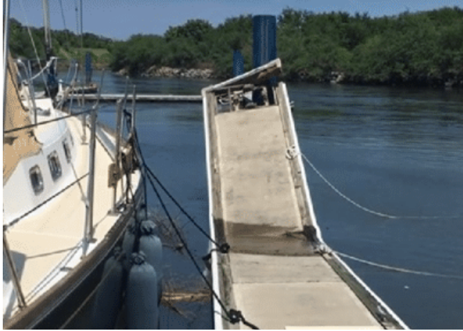
Figure 34: Docks lifted off pilings due to extreme water level changes.
