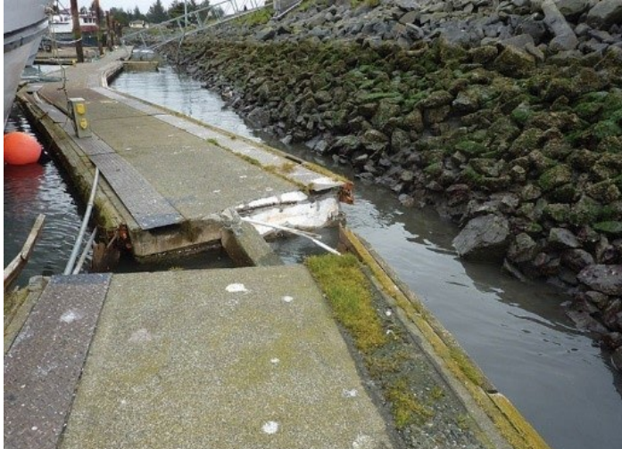
Figure 46: Broken dock in California from tsunami waves.
