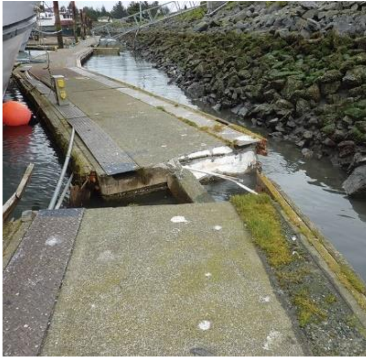
Figure 36: Broken dock in California from tsunami waves.
