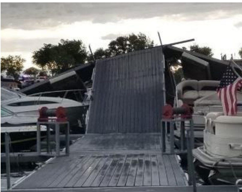
Figure 34: Docks lifted off pilings due to extreme water level changes.
