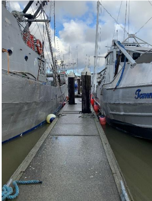
Figure 35: Newer strong pilings at Squalicum Harbor may prove of insufficient height to anchor docks during tsunami inundation.
