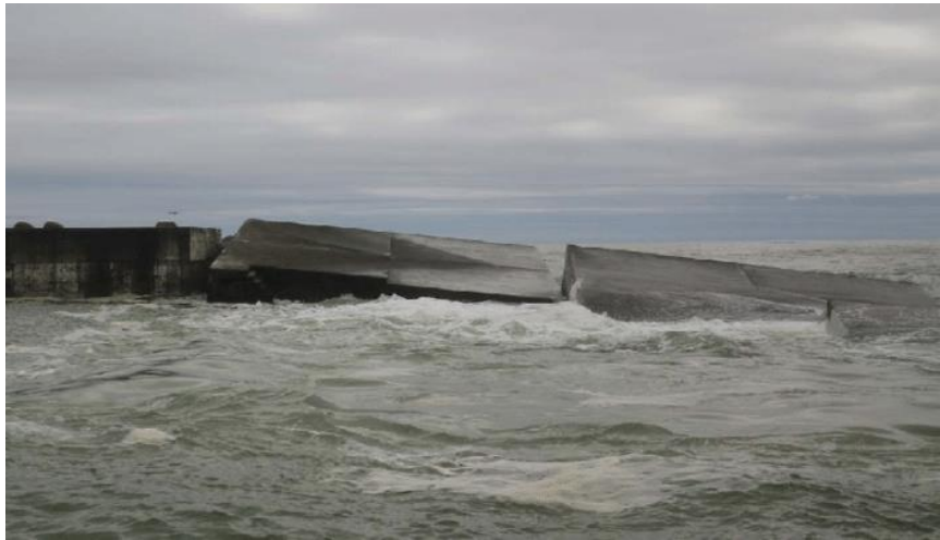
Figure 42: Breakwater failure in Japan after 2011 Tohoku Tsunami.
