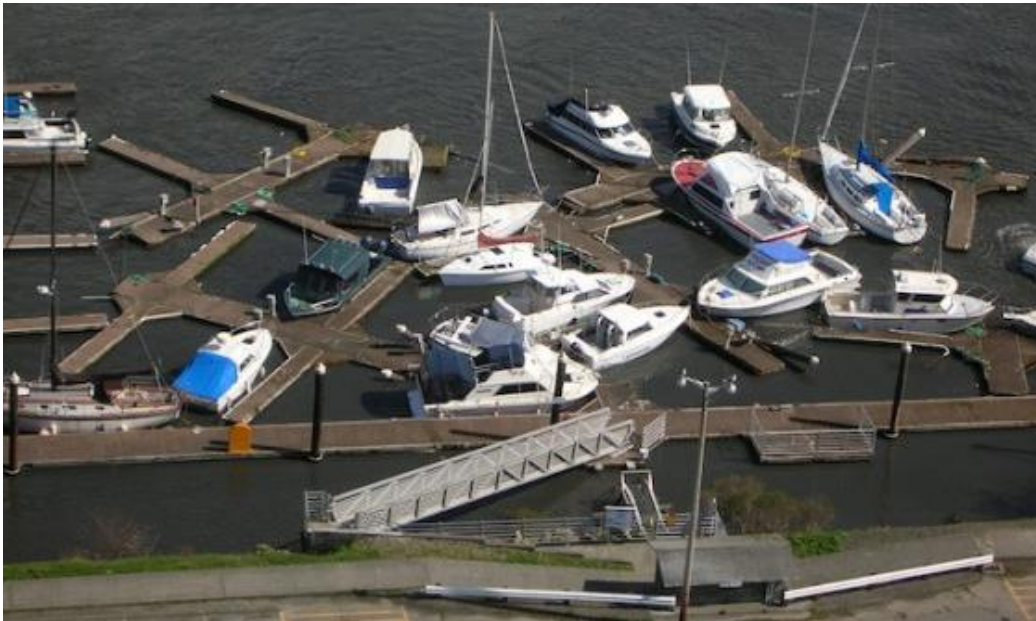
Figure 6: Docks broken from Japan 2011 distant tsunami event in Brookings, OR. USCG Photo by Group Air Station North Bend
