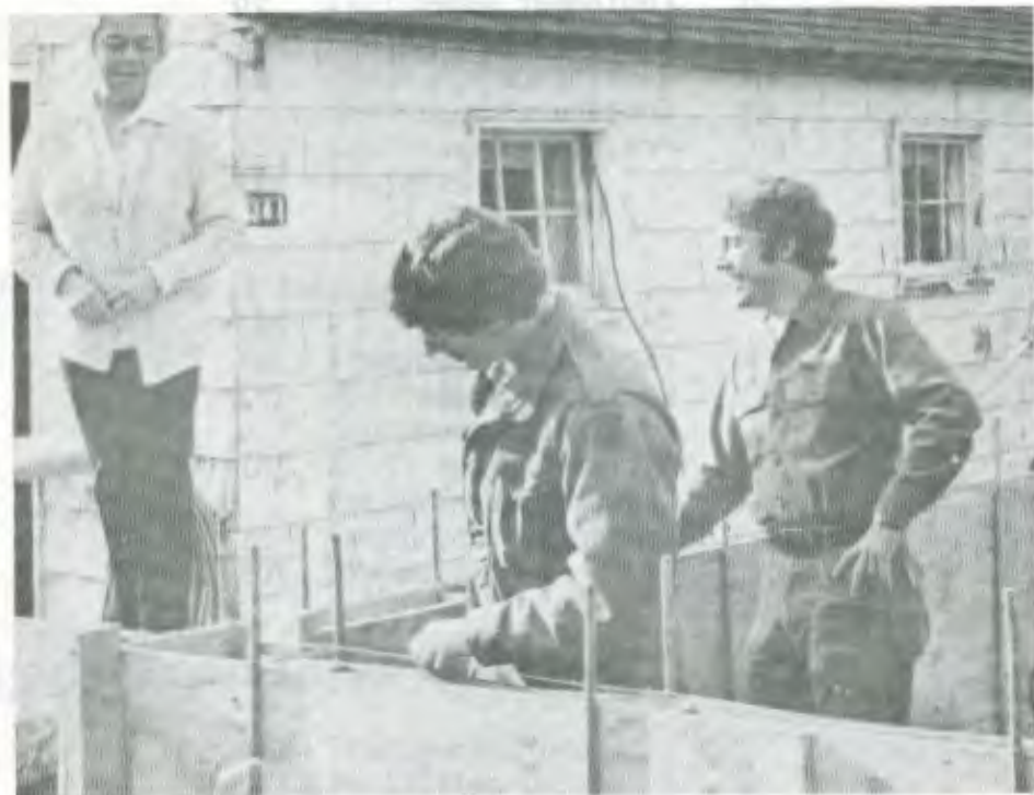
81st Infantry Brigade personnel constructing a home for a widow in Seattle who had become destitute. The garage in the background is her current home. This project was undertaken as part of the National Guard's concern for community assistance.
