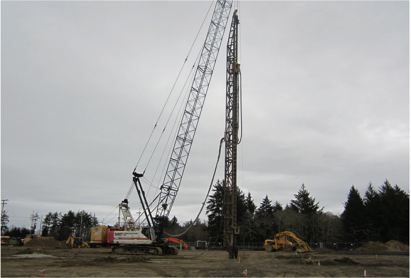
Drilling rig preparing to install one of 160 piles for the Ocosta Elementary School. Photo Credit: Degenkolb Engineers
