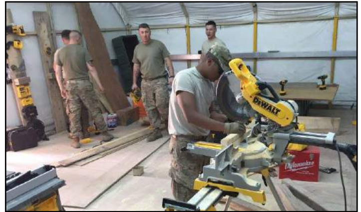
Soldiers from the 176th Engineer Company perform construction operations at Camp Arifjan, Kuwait in July 2016. The Snohomish based unit deployed in early 2016 in support of Central Command's mission in the Middle East.
