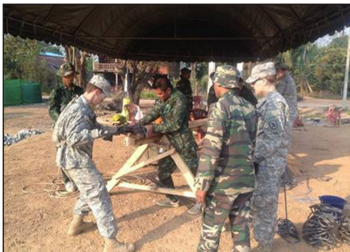
Guardsmen from the 176th Engineer Co. work with the Royal Thai Army on a new schoolhouse in the Ban Sa la Kai Fub School in Sukothai province, Kingdom of Thailand. The project was completed and is now open for children to use.
