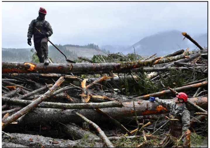
Tech. Sgt. Tayler Bates and Tech Sgt. Tony Rohrenbach, members of the Washington Air National Guard 141 Civil Engineer Squadron discuss how to remove debris to drain the water from their search area. (U.S. Army photo by Staff Sgt. Rory Featherston WA ANG)
