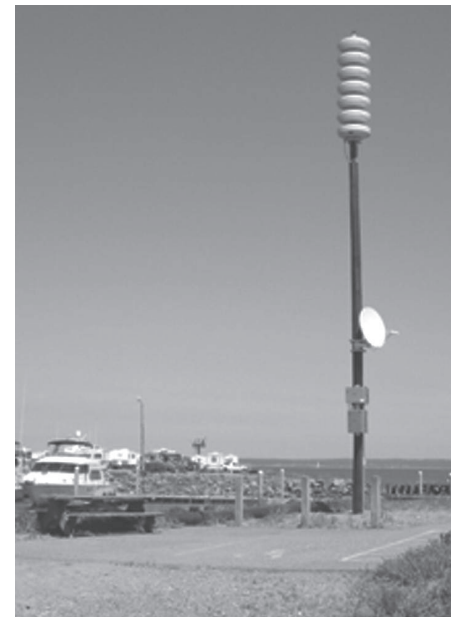
Point Hudson "All Hazards Alert Broadcast" (AHAB) unit is one of many sirens installed in Clallam and Jefferson counties. AHABs can be activated by satellite from the State Emergency Operations Center or by radio from local Emergency Operation Centers.
