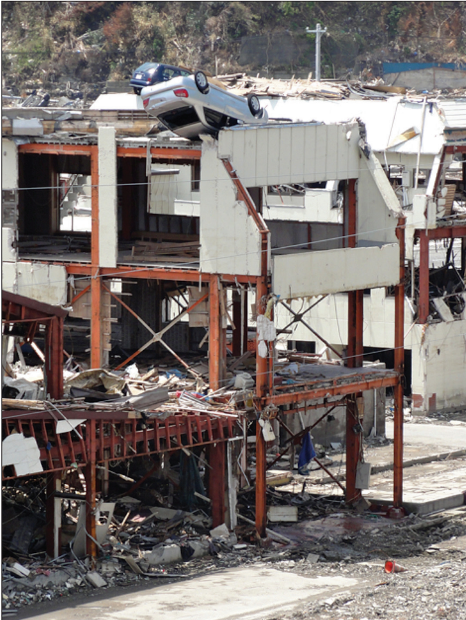
Onagawa, Japan, March 2011. During the tsunami, cars were deposited on the fourth floor roof of building. Credit / Laura Kong, IITC
