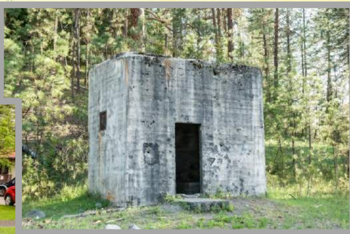
Pump House at Camp Seven Mile: belongs to 22 features at a former CCC camp that are eligible for NRHP listing
